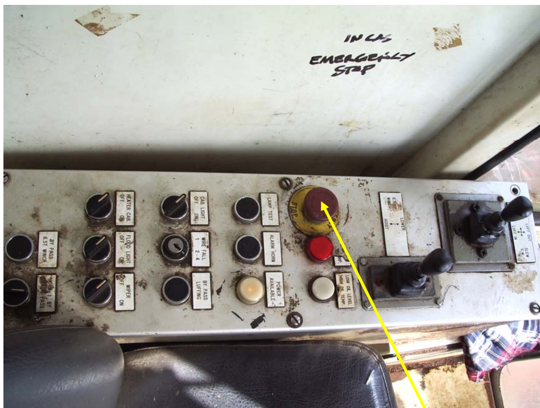
No. 1 crane controls showing emergency button.
