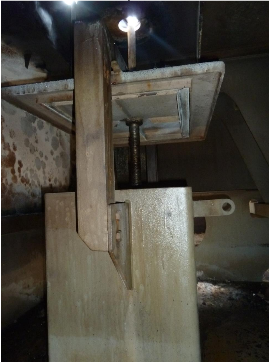
Supply fan ventilation trunking inlet
