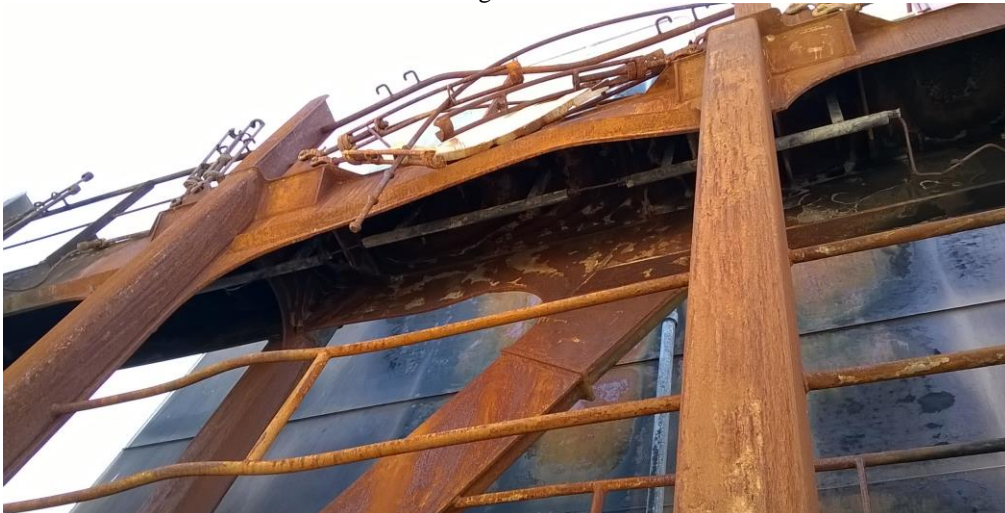
Damage to lashing bridge
