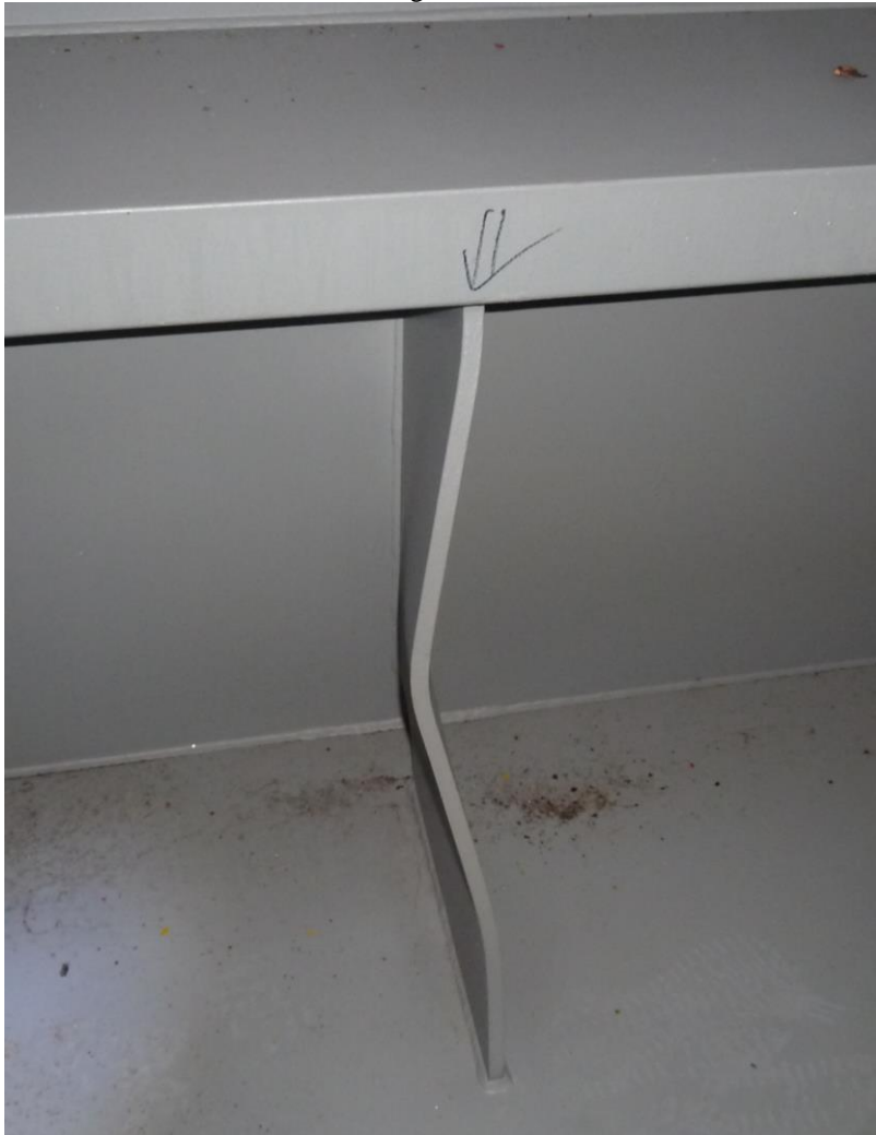
Brackets on stringer deformed
