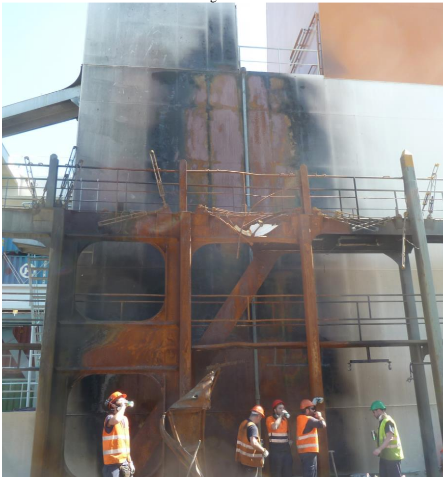
Damage to the lashing bridge in the foreground and to ER casing fwd bulkhead behind
