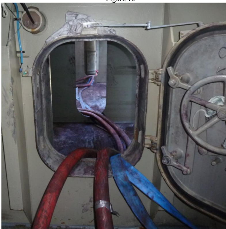
WT door (frs 59-60) from stbd side deck 2 underdeck passageway, looking through to CH 9
