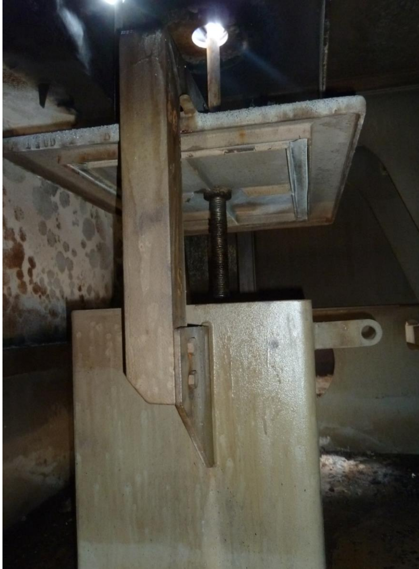
Example of the screw down ventilation trunking lid arrangement situated directly below X deck walkway
