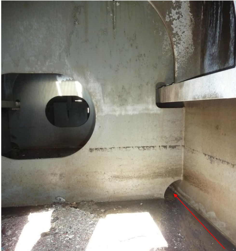
Space directly below X deck where vent trunking inlets are situated showing small drainage cut-outs on floor for normal drainage of this space (upper deck).
