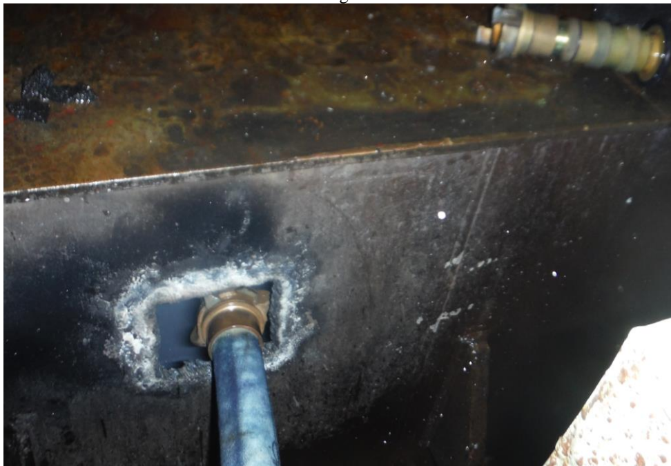
Cooling hose in cut-out
