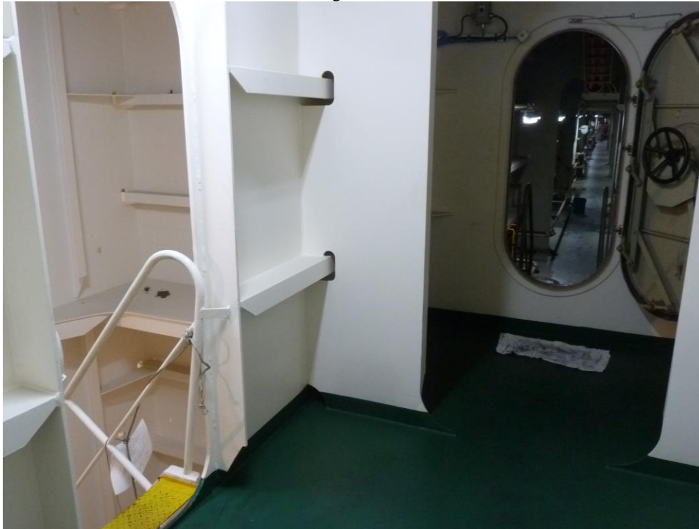
Aft WT door (fr 12) at the end of the stbd deck 2 passageway, water flooded above this level and down the stairwell in the foreground into the steering gear compartment.
