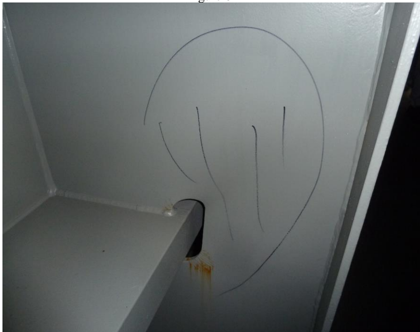
Deformation on vertical girder
