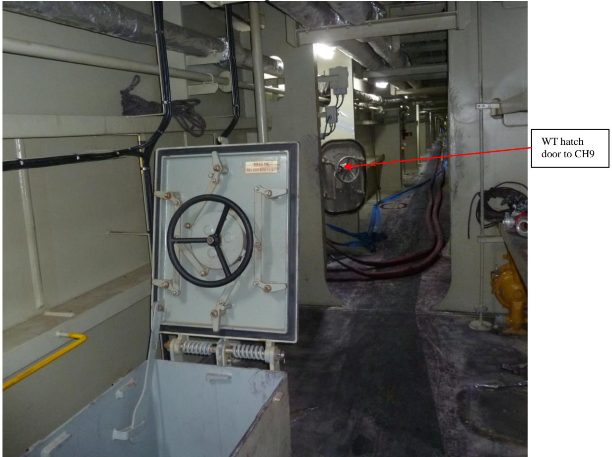
Raised access hatch to stbd bunker station (frs 55-56) in foreground and further behind can be seen the open WT hatch door (frs 59-60) to CH 9.
