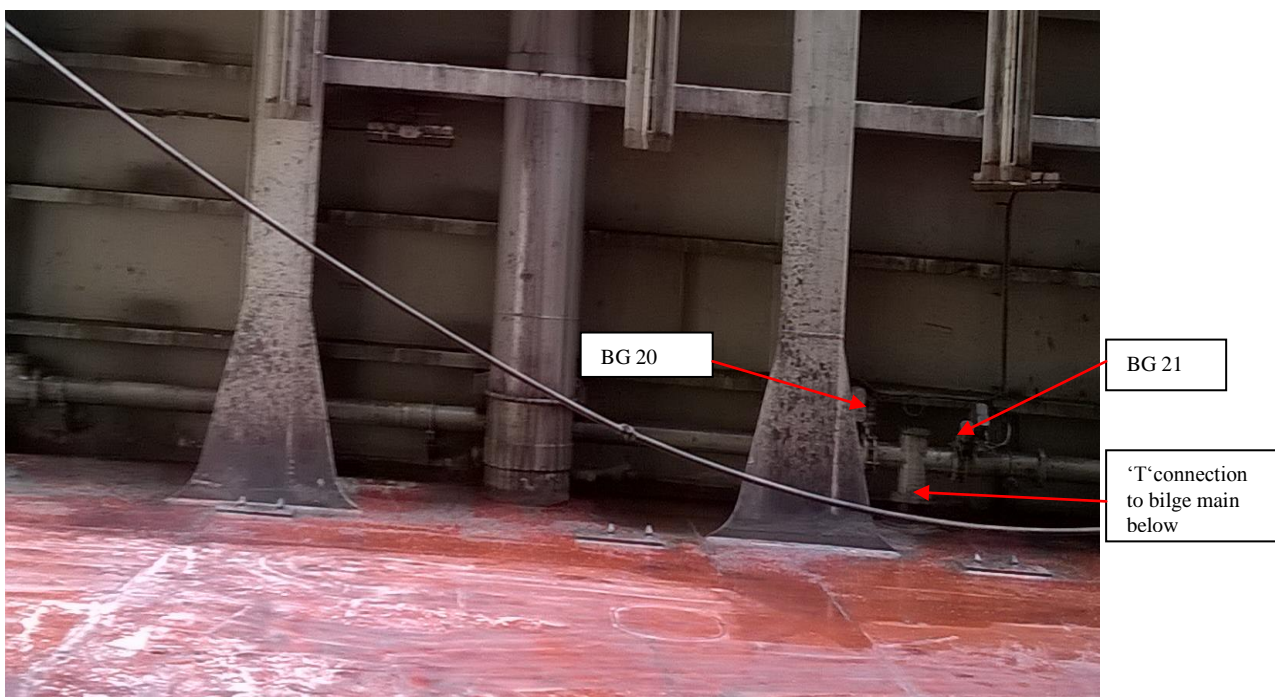
Port and stbd bilge lines arrangement dropping down to bilge main in duct keel below tank top.
