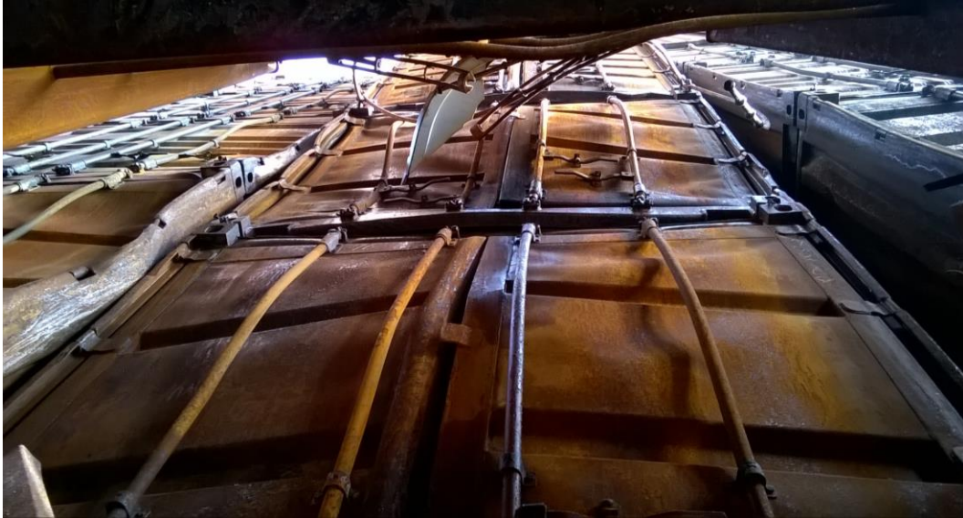
Damage to containers above and surrounding 700582
