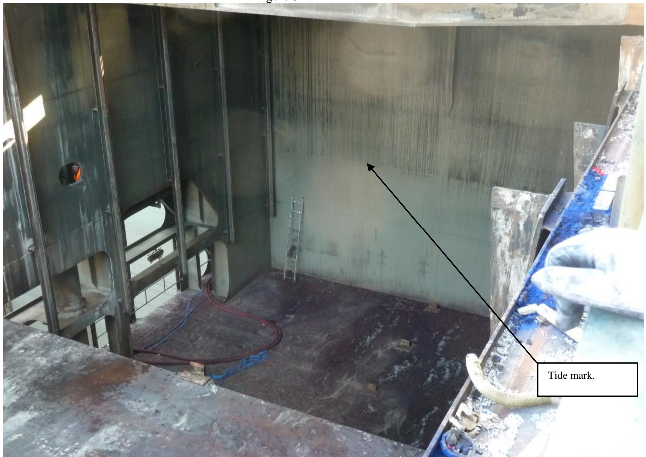
Tide mark clearly seen above ladder on deck 2.
