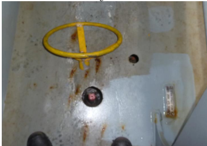
Portable handwheel for operating the ventilation trunking lid. The end of operating spindle can be seen (red end) as can the opening for the position indicating tale rod
