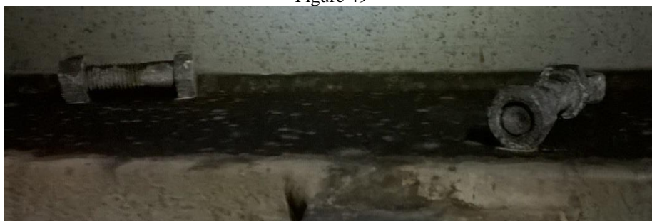
Missing nuts and bolts on framing below
