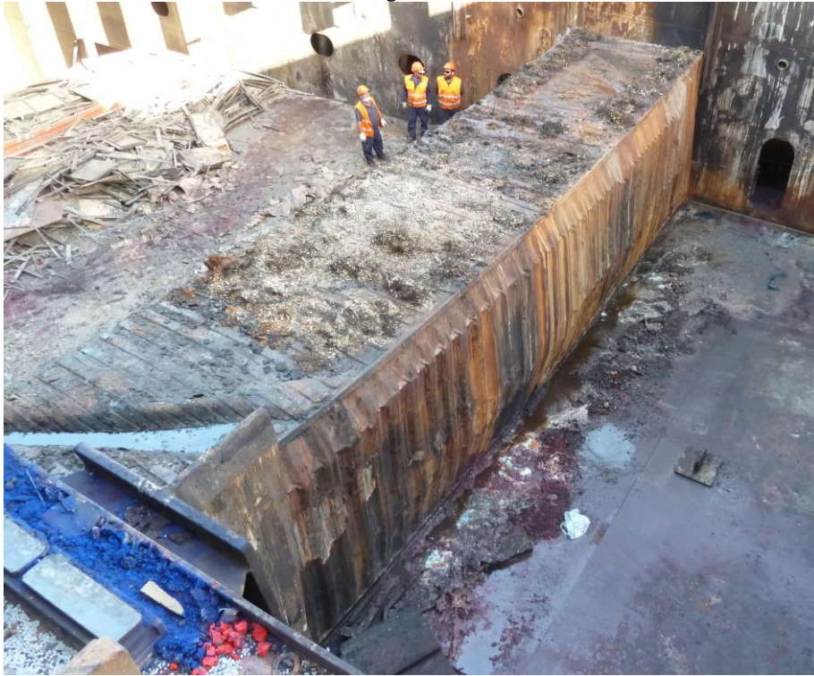
Container 700020 showing deformation on outboard side
