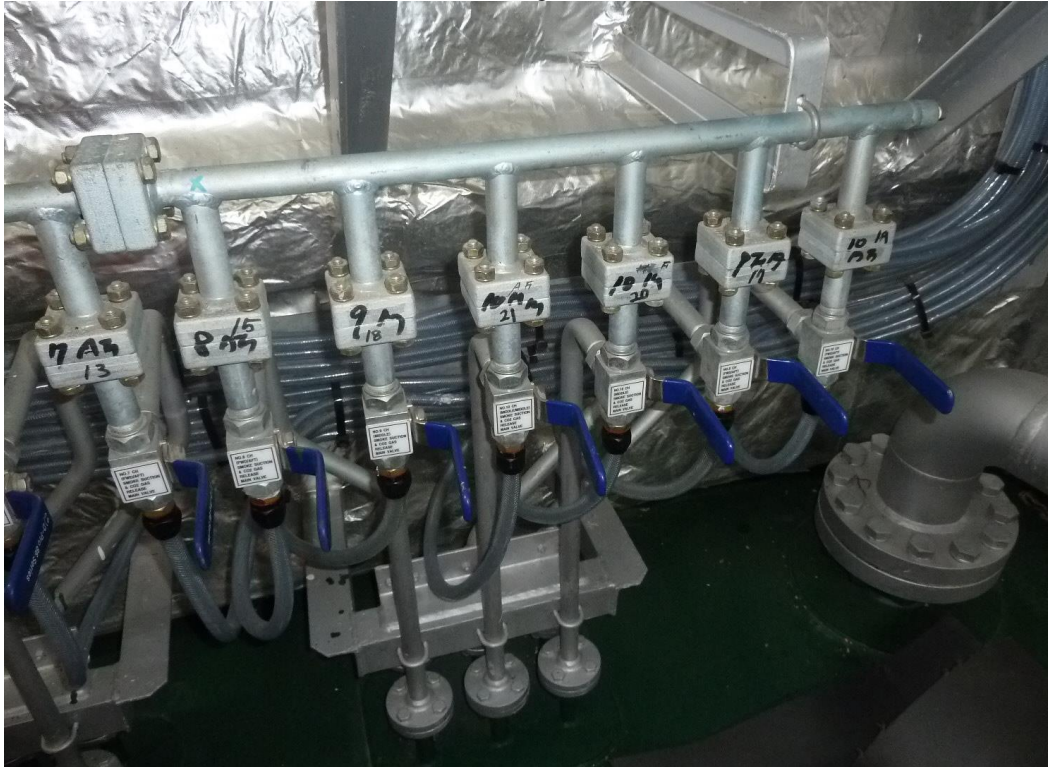
Section of CO 2 distribution manifold showing blue handled levers used to change over from smoke sampling to CO 2 delivery
