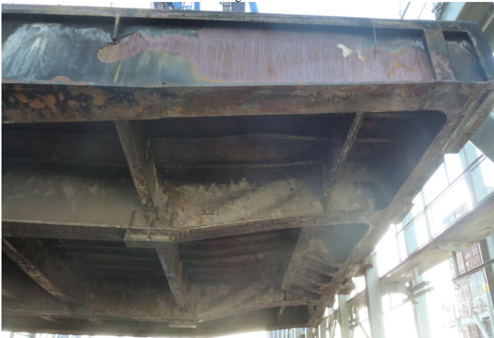
Bay 70 stbd inner hatch cover showing deformation due to heat damage
