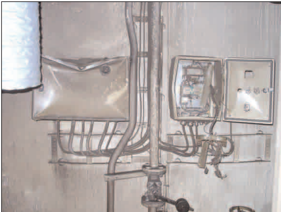
Damage in bow thruster room
