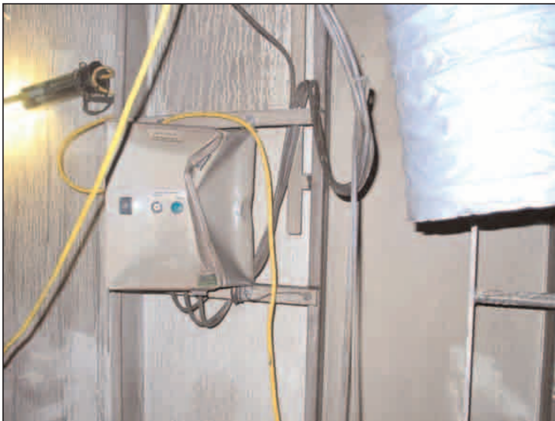
Damage in bow thruster room
