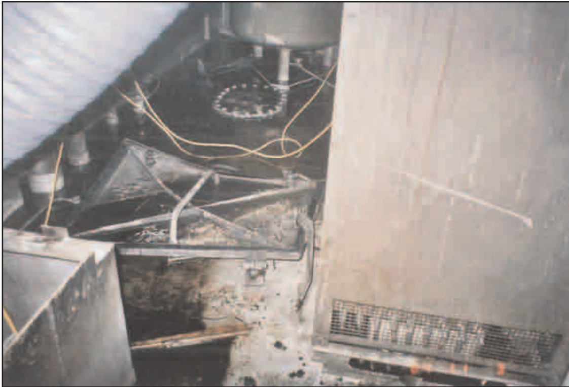
Damage to hatch
