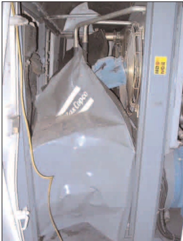
Pressure damage to compressor enclosure
