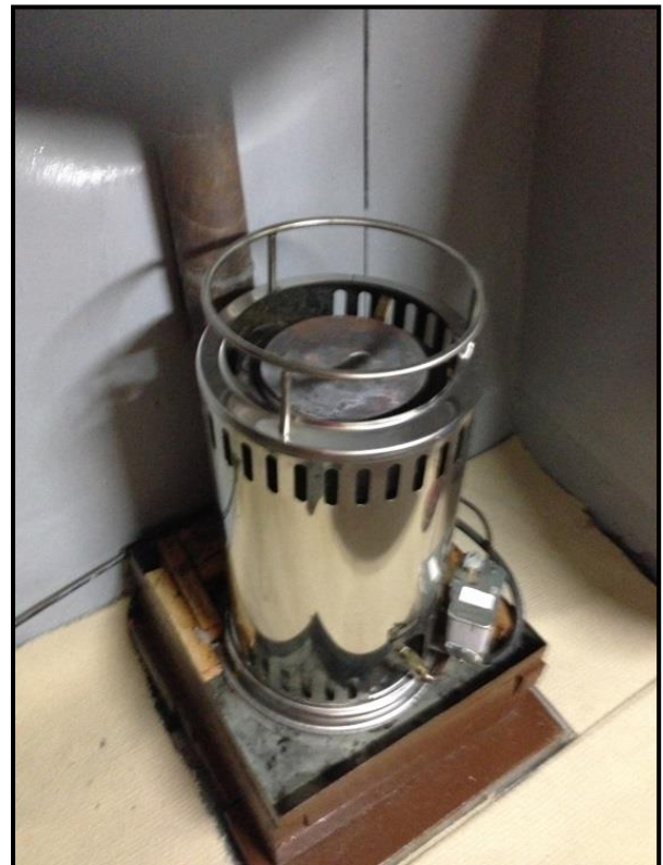
The oil stove, picture was taken in June 2018
