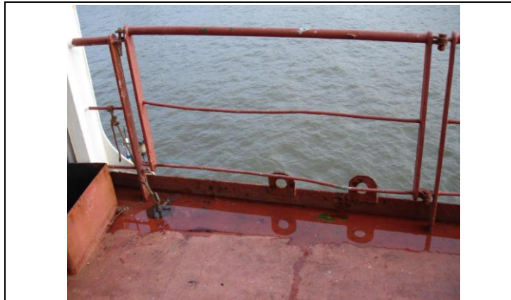
A photograph of the aft starboard hinged rail section showing deformation reportedly caused by the loose pallet
