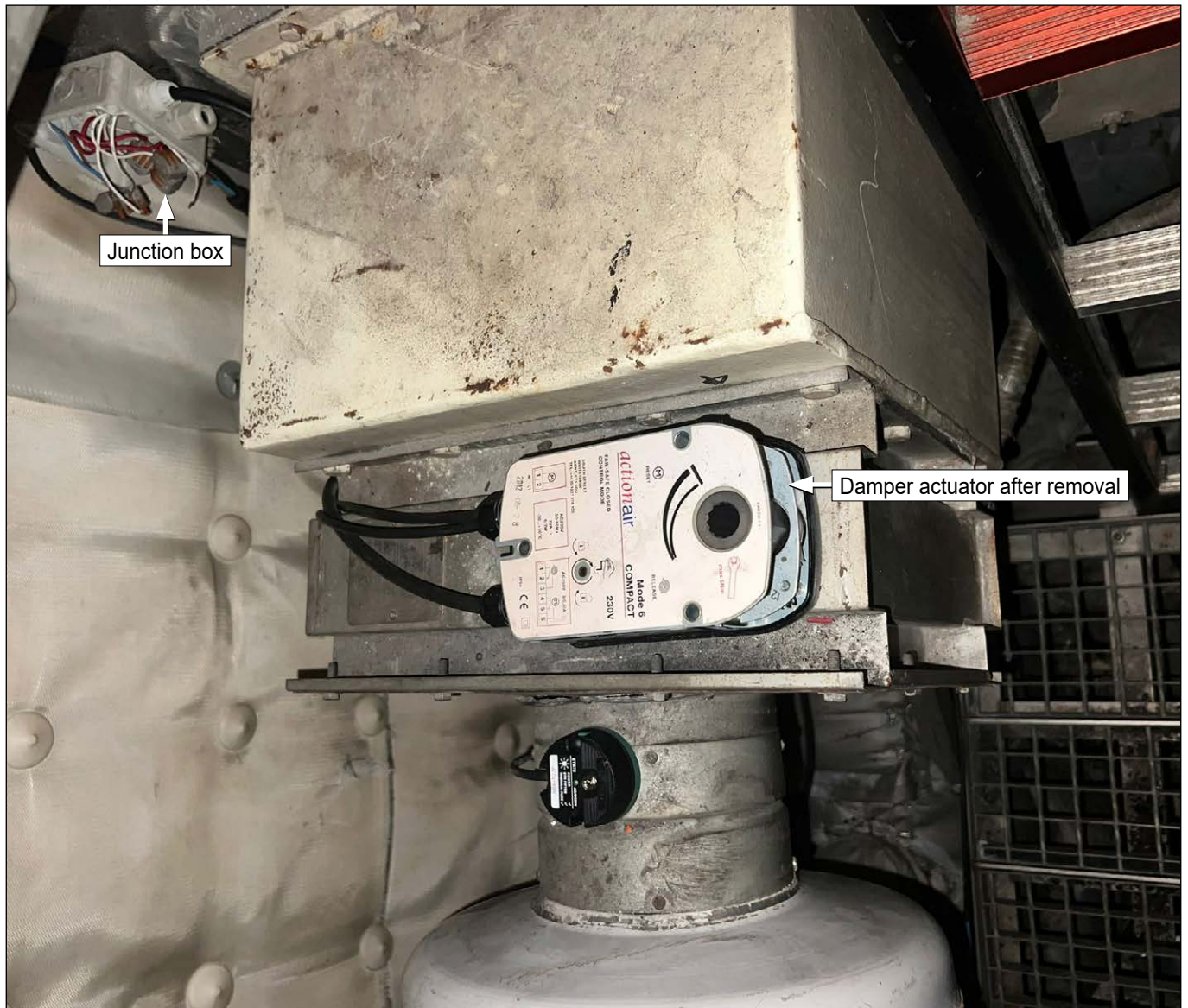
Figure 3: Removed damper actuator and junction box showing the wiring
