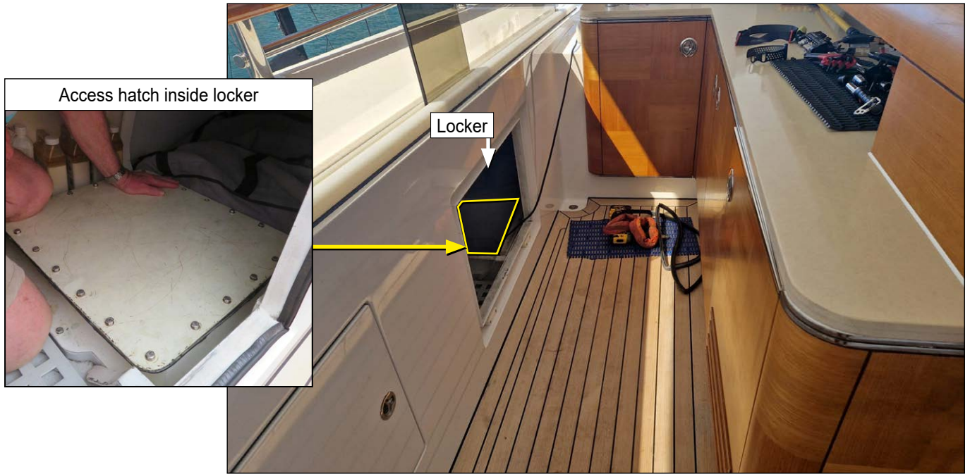
Figure 2: Access to overpressure duct compartment
