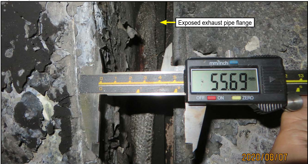
Figure 21: AE2 gaps in heat shields and exposed exhaust flange
