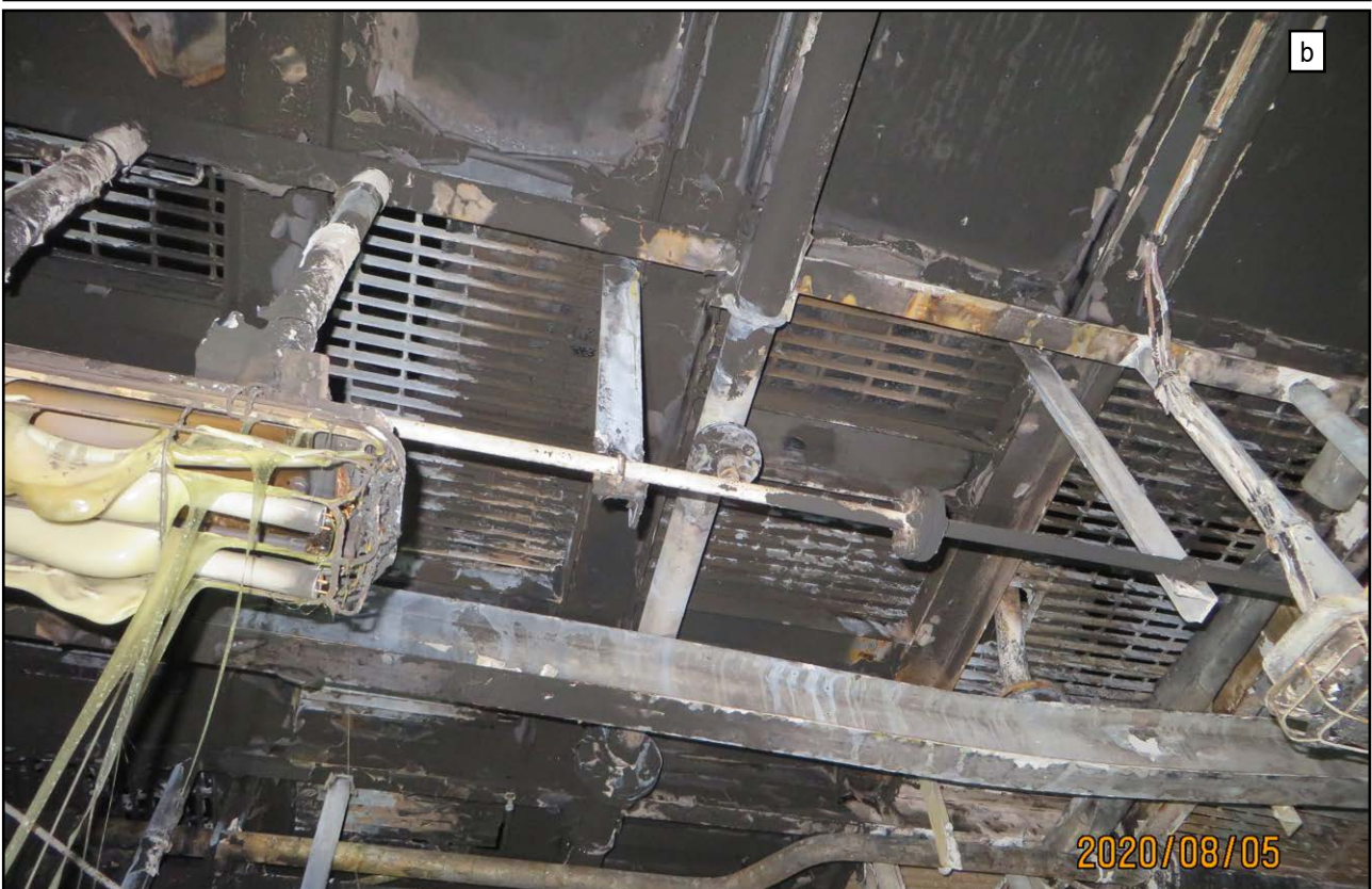
Figure 23: Boiler platform fire damage (a) and view up to boiler platform from auxiliary engines (b)
